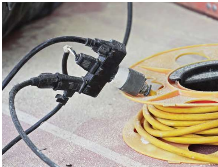
Figure 2-17. Damaged power cord and overloaded extension cord.
