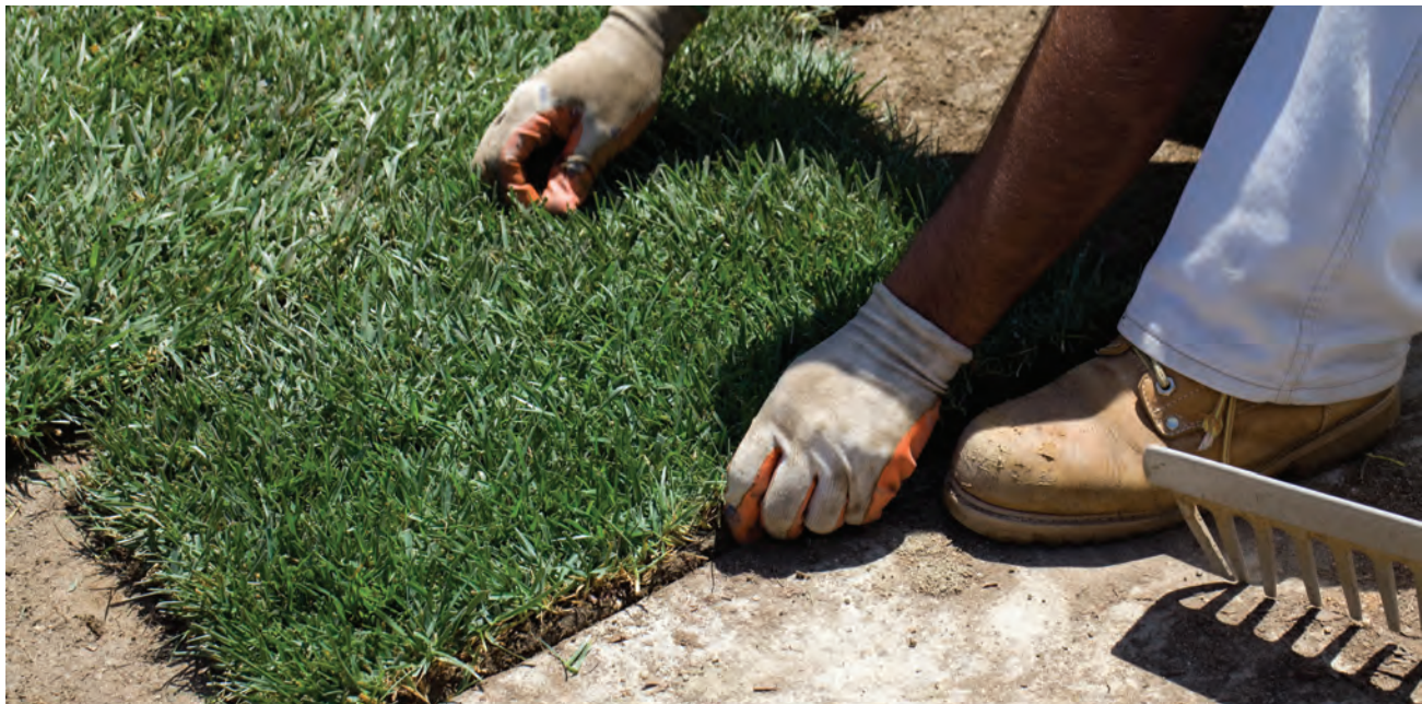
Figure 14-5. Installing sod in a staggered brick pattern where the finish grade is slightly below the sidewalk.
