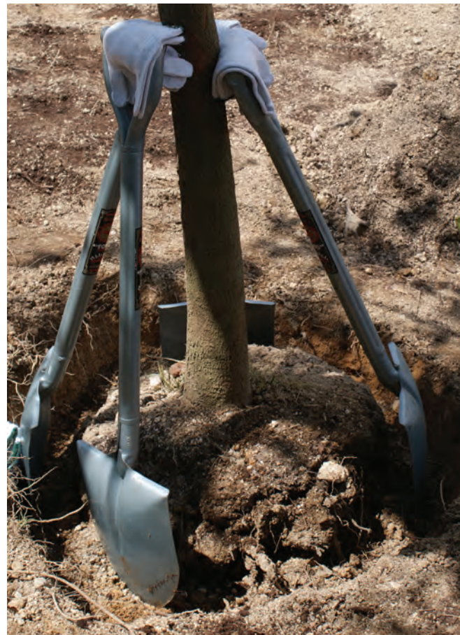
Figure 13-22. Tree placed in a wide, shallow hole with the flare slightly above existing grade. Backfill soil will be slightly firmed and a catch basin constructed surrounding the root ball. Mulching and watering will complete the task.
