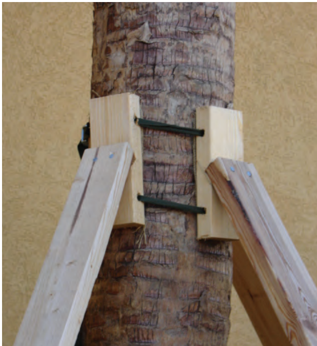
Figure 13-27. Close up of palm banding and bracing technique. Note: Burlap should be placed beneath the wood battens as a precaution against trunk scarring.
