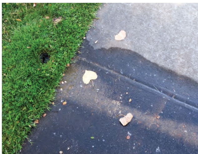
Figure 10-23. Leaking popup sprinkler head.
