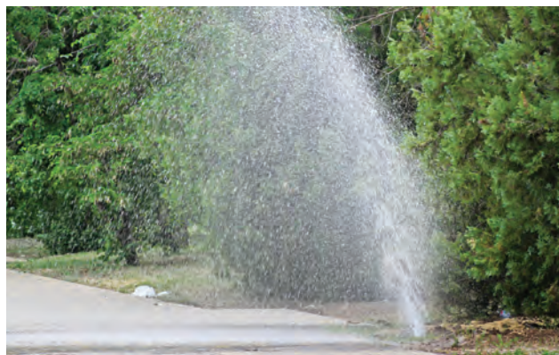
Figure 10-24. Broken irrigation pipe.
