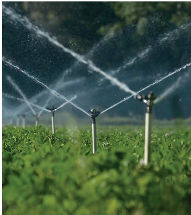
Figure 8. Overhead irrigation system in nursery production.
